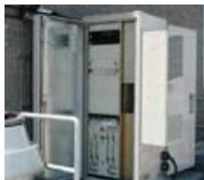
DVB-H Base Station
