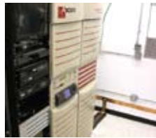
State College Transmitter Site
