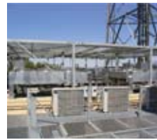
Community Heat Exchanger
